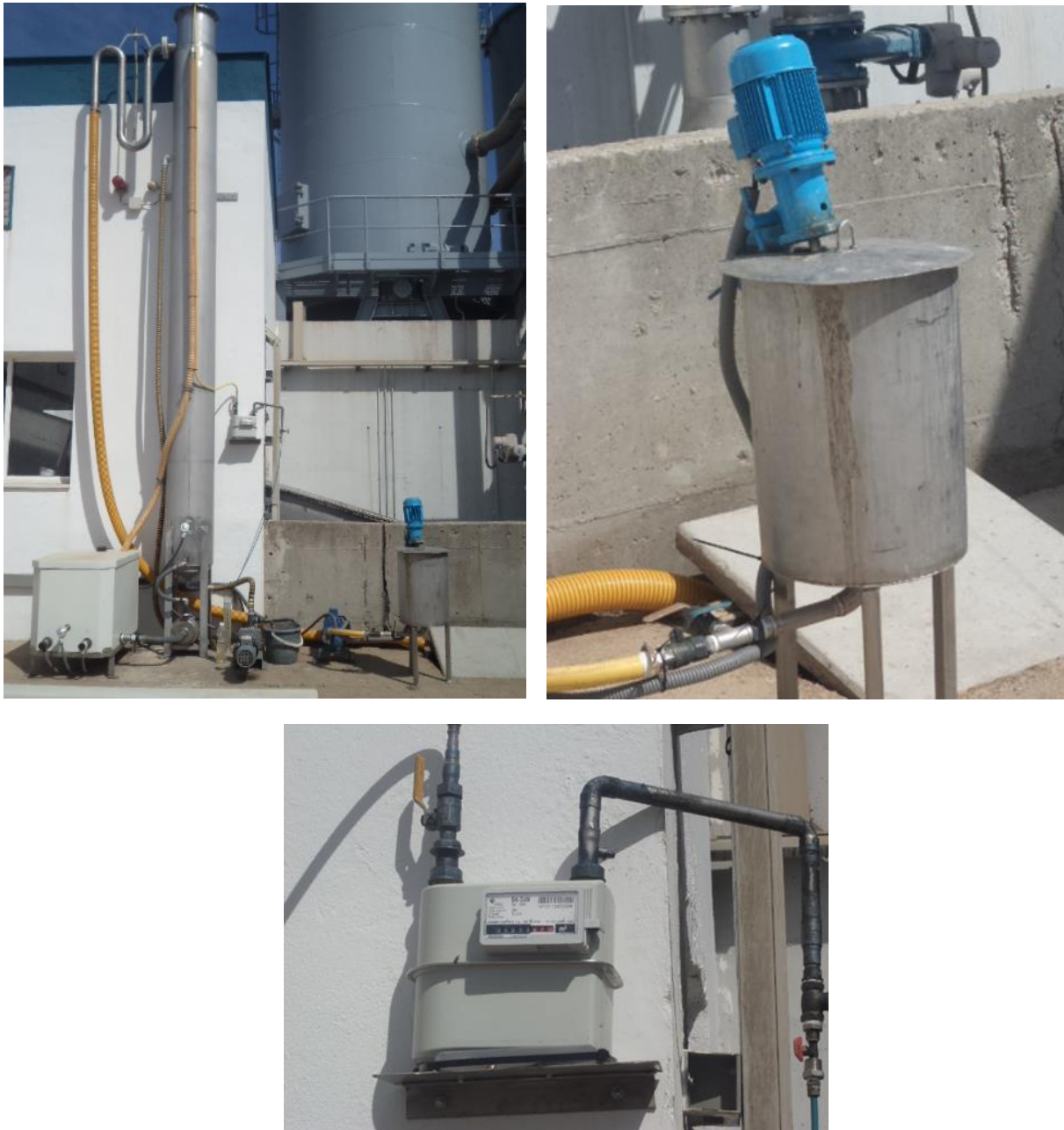
Image 5. Co-digestion Pilot Plant overview, feed tank and gas flow meter from EMASESA.
