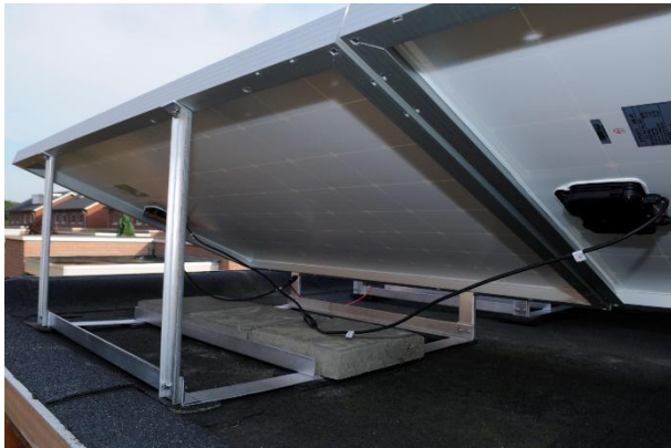
Fig. 5: An example of how new concrete paving slabs are being used as ballast for a photovoltaic flat roof system.
