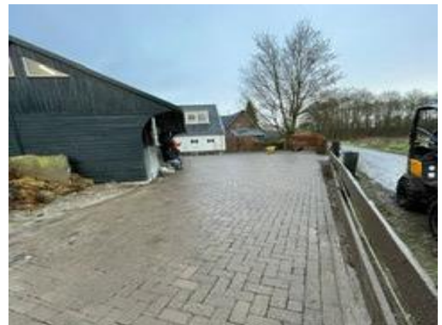
Fig. 8: Concrete pavers were being reused at the different farms nearby the renovation project.
