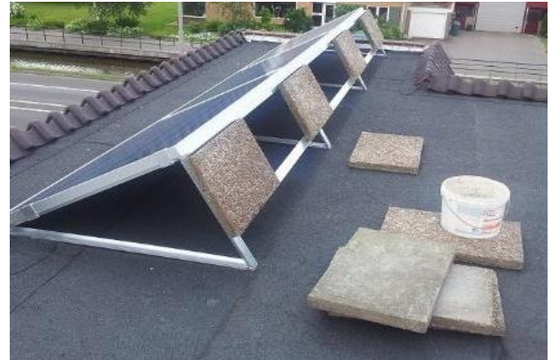
Fig. 6: An example of how concrete paving slabs can be reused as ballast for a photovoltaic flat roof system.
