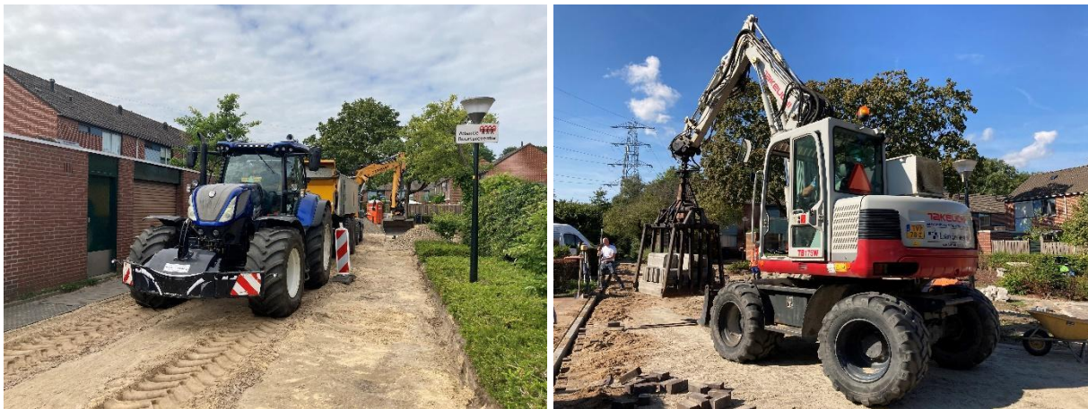
Figure 8. Tractor with tipper and in the back an excavator at Griffiersveld in July 2022 (by courtesy of Bram Entrop). Figure 9. A crane transporting kerb stones at Griffiersveld in September 2022 (by courtesy of Lisanne Hagen).
