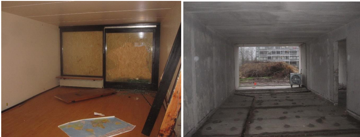
Figure 5 - Demolition of exposed residential building in Gellerupparken, Aarhus, 2015. The building is total stripped for interior materials and cleansed for contamination of PCB before demolition. After crushing on site all concrete materials are recycled and sold by the contractor.
