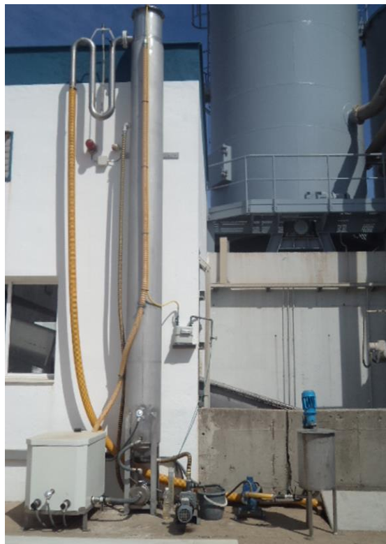
Figure 29. General view of the pilot plant in EMASESA facilities.
