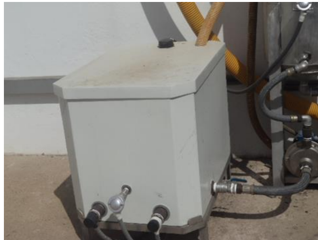
Figure 30. Tank with resistors
